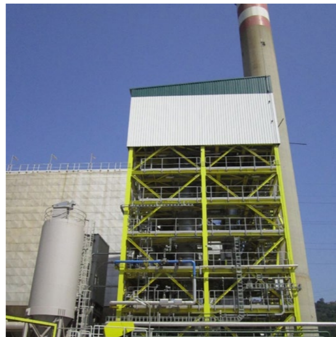
Calcium Looping 1.7 MW demo plant completed in La Pereda, Spain. The pilot plant was commissioned in 2012 with demonstrated capture efficiency of over 90%
